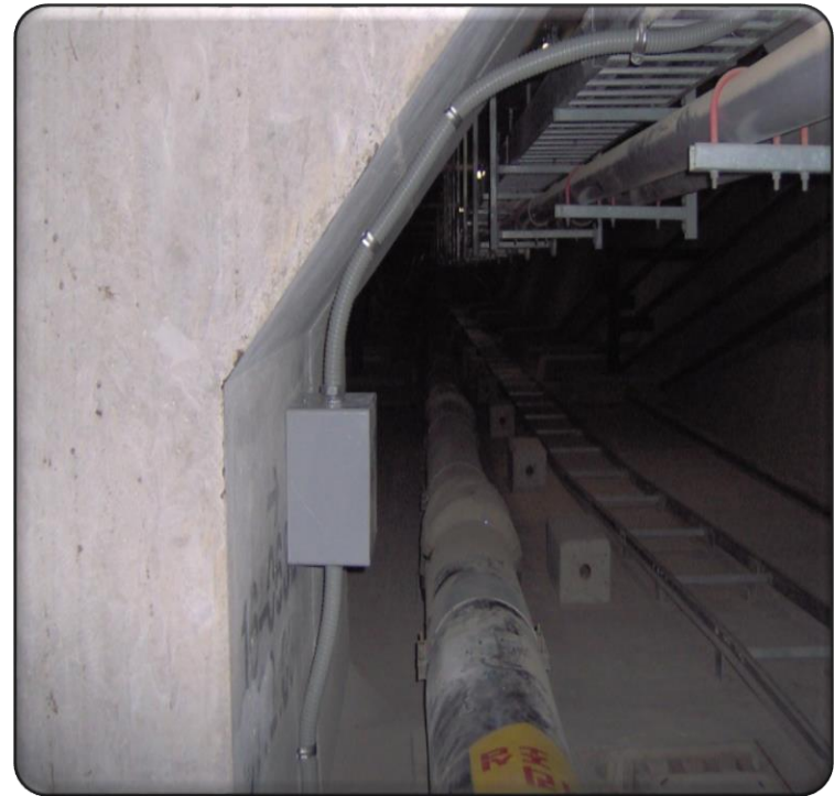
Pull Box for Work Process
